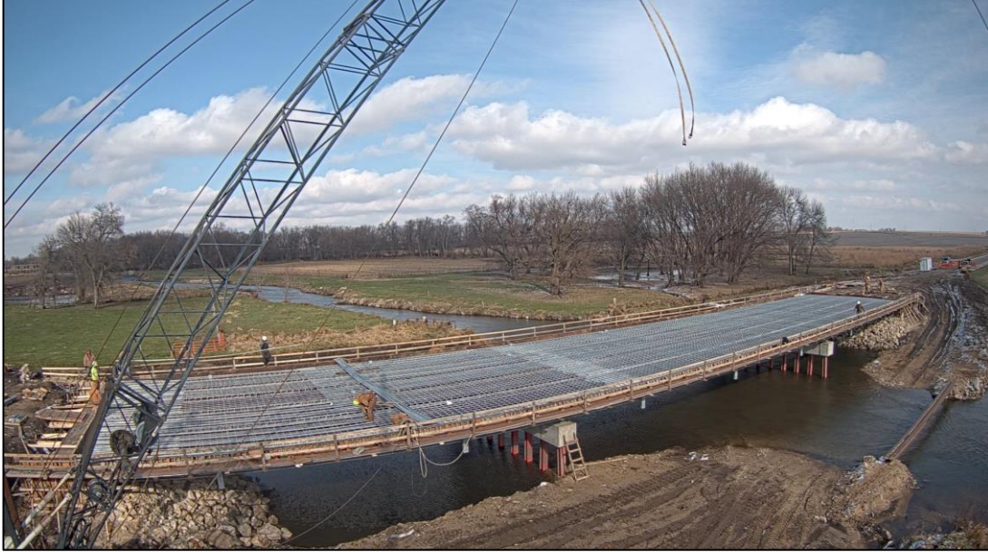
Figure 5. First bridge constructed with CGR, using 75 tons: Buffalo Creek Bridge in Independence, Iowa, USA (Source: AZZ Metal Coatings)
